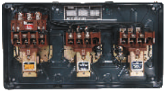
Interior View of MK2 SASD
