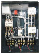
Interior View of MU-G30W FASD
