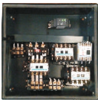
Interior View of MU-G20W FASD
