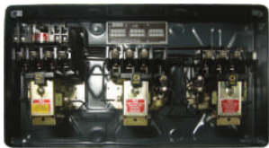
Interior View of MK1 SASD
